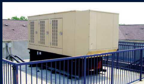
Full backup generator for all power
