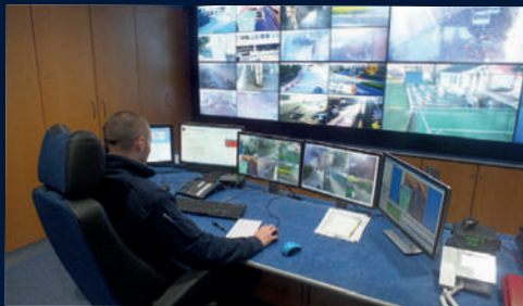
Security Control Room
